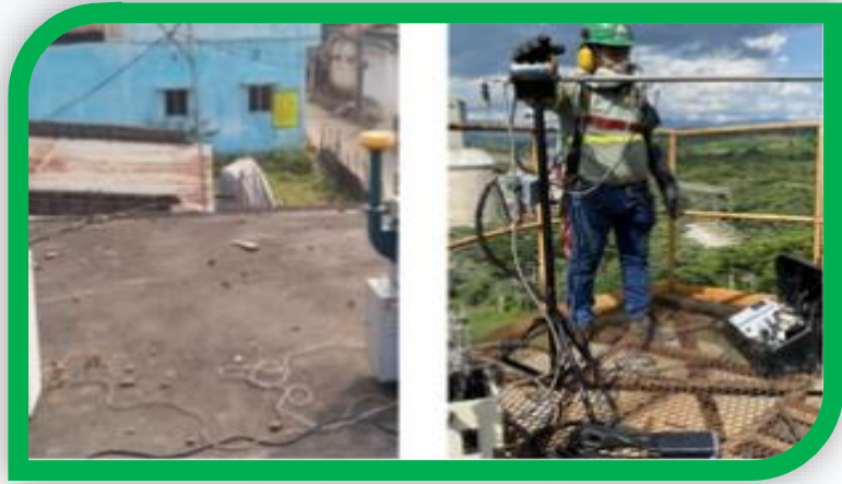
Industrial Air Quality Monitoring
